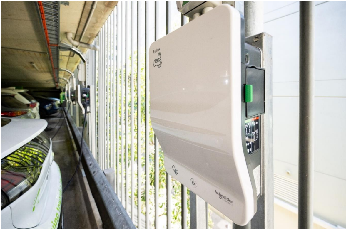
Figure 3: EVlink Smart Wallbox Chargers (7.4kW – T2 – RFID) installed at Wyatt UPark
