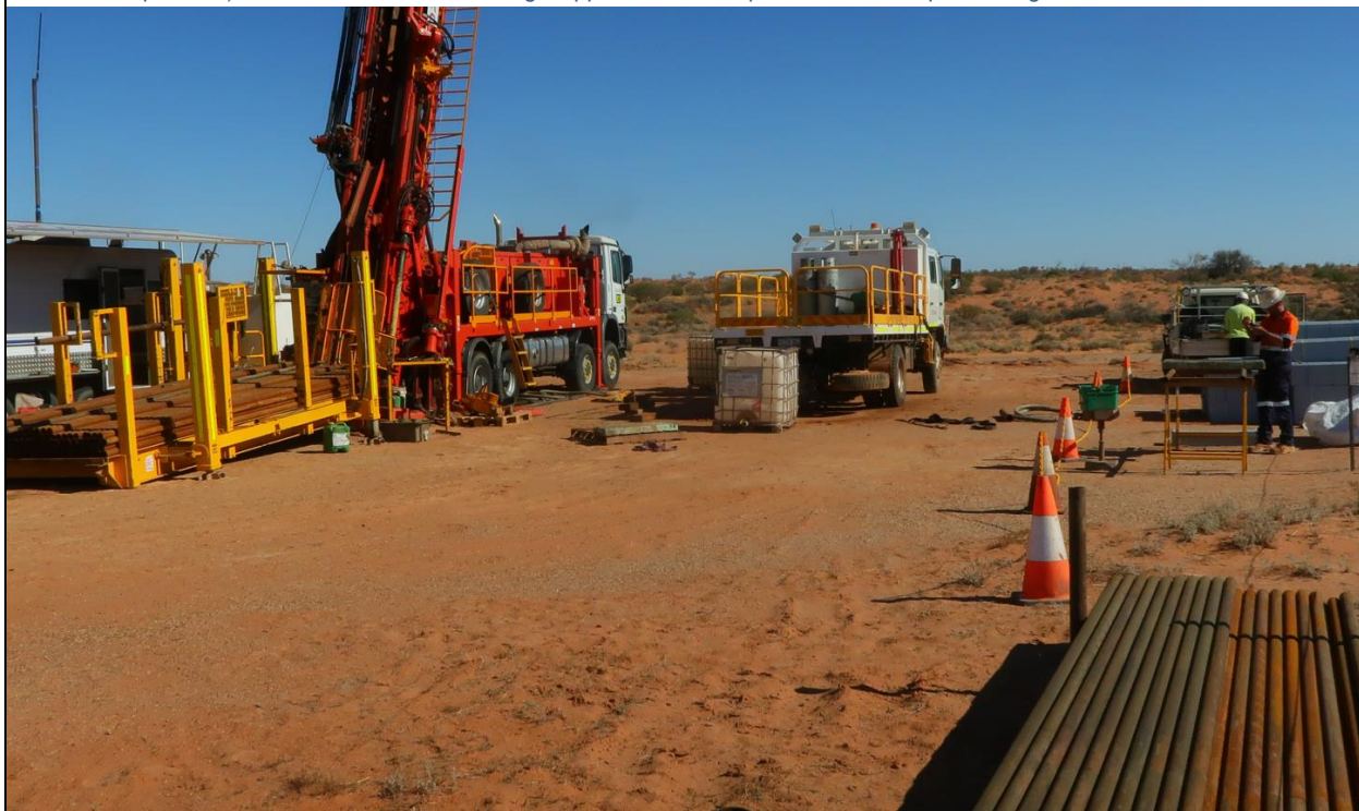
Figure 6. An example of the 50x50m drill pad with the drill rig (left) and core processing area (right). The photograph of typical drill site showing (L to R) rod rack/sloop (on a hydraulic powered flatbed truck platform), driller office caravan, drill rig, support truck, core presentation and processing area.
