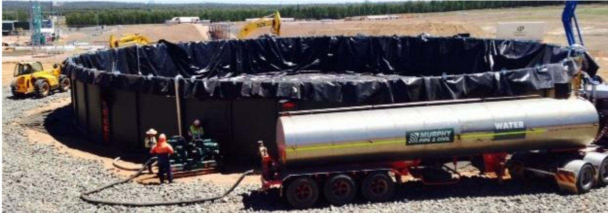
Plate 3-2: Example of above-ground storage tank. Source: Tango Hire 5
