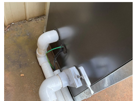
Photographs show incorrect depth of burial, lack of mechanical protection and incorrect wiring system (conduit) has been used.
