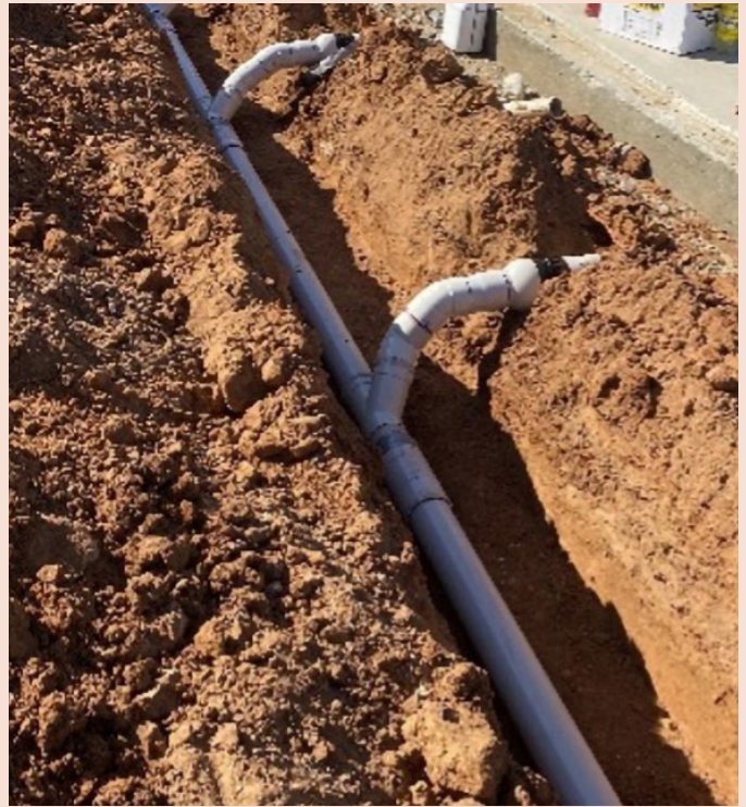
This photo demonstrates an acceptable visible base of trench with a completed installation ready for inspection.
