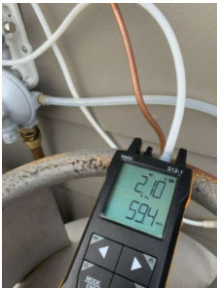
Image shows Integral 2-stage regulator not commissioned, the outlet pressure at the regulator is set at 2.1kPa
