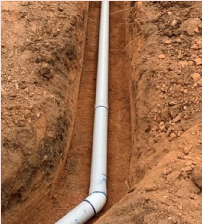
This photo demonstrates a section of sanitary drainage laid on a compliant and visible base of trench ready for inspection.
