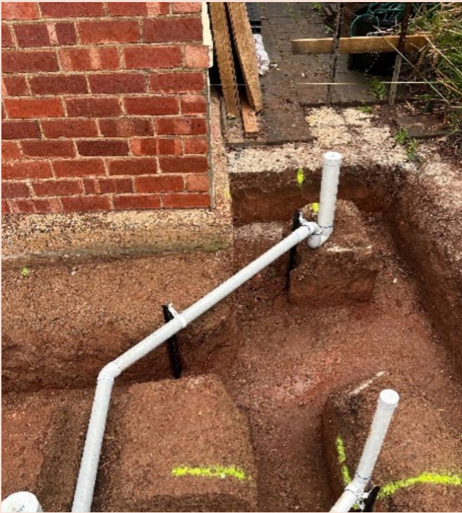
This photo demonstrates star picket pipe supports that have been installed for branches located within footings. Lagging is to be installed around pipes, fittings and joints after hydrostatic testing has confirmed there are no leaks after the inspection.
