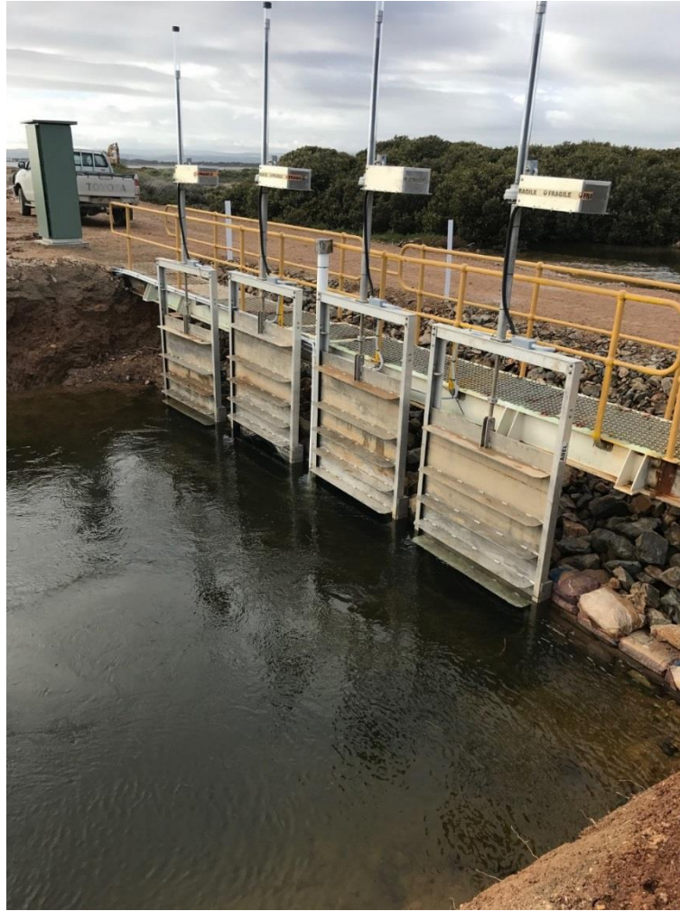
Figure 10 Tidal gate infrastructure installed in the seaward levee bank of Pond XB8A at the Dry Creek salt fields
