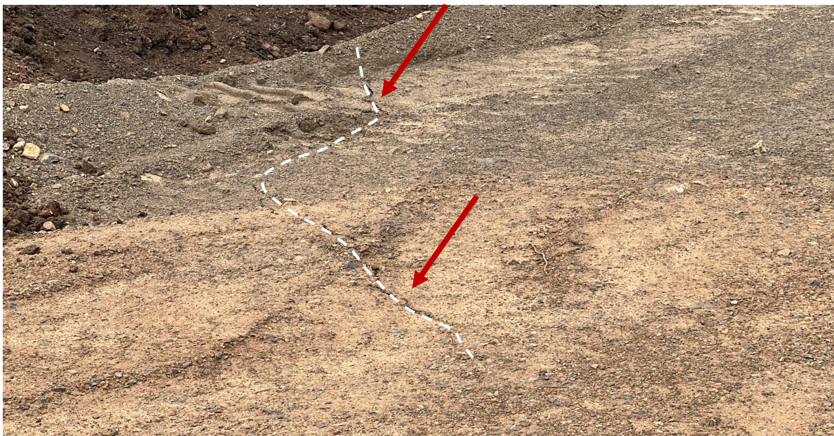
Figure 11: Cracks observed in recent lift material placement.
