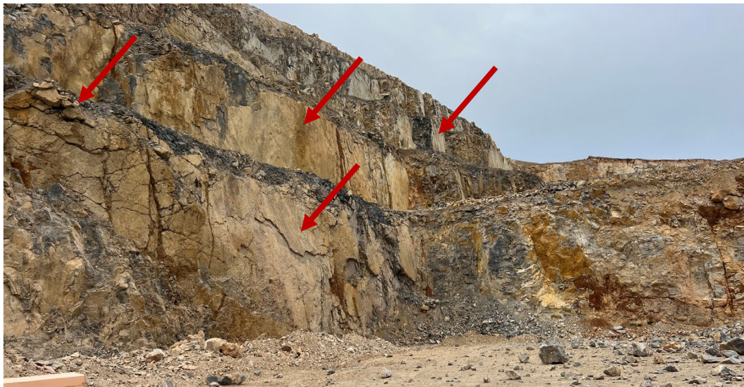
Figure 13: Highwall of the southernmost end of the pit displaying crest damage sliding potential.
