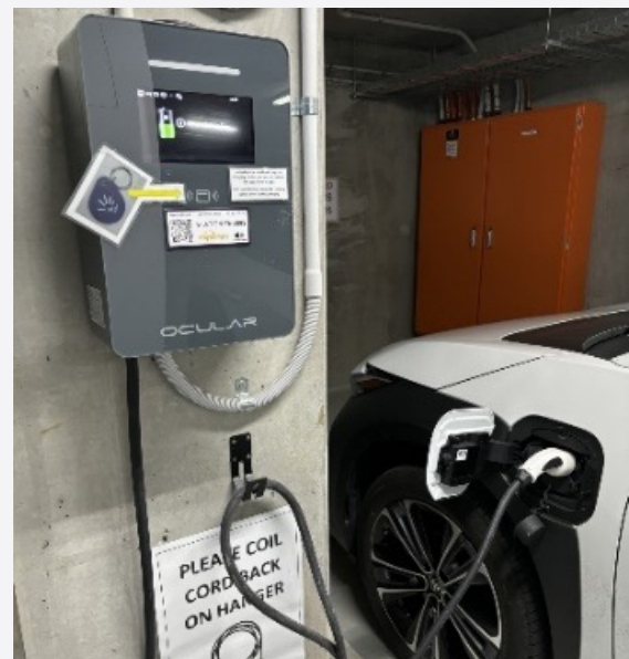
Charger 2 installed at Uniting Communities
