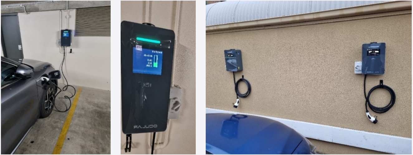
Images 3.10 (b): Showing the images of installed chargers at Centacare locations Wakefield Street & Grange Road
