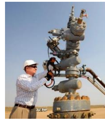
Premier Weatherill turns the valve to kick off gas production from Santos JV Moomba 191 in 2012
