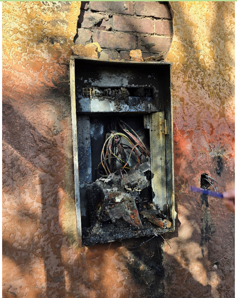
Photograph shows where fire has originated at the switchboard and has spread through to the dwelling, as openings weren't sealed.
