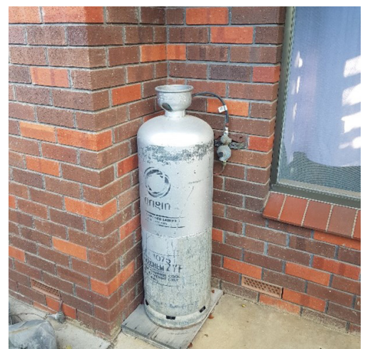
Non-compliant regulator location, regulator too low.
