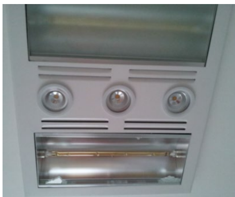
Figure E 11: Example of an electrical product failure
